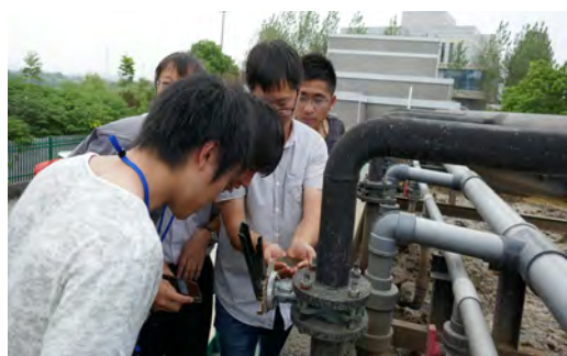
農村ため池の浄化施設現場 The site of water purification facility for a rural village pond
