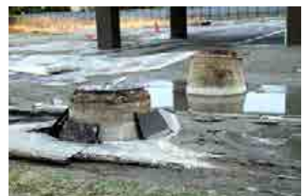
Liquefaction phenomenon (High groundwater level)
