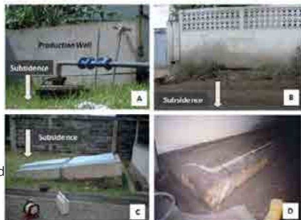
Impacts of Land Subsidence
